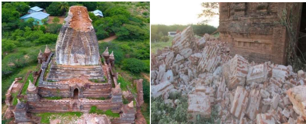
Figure (33) Damages in Repaired Parts and Upper Part of Monuments
