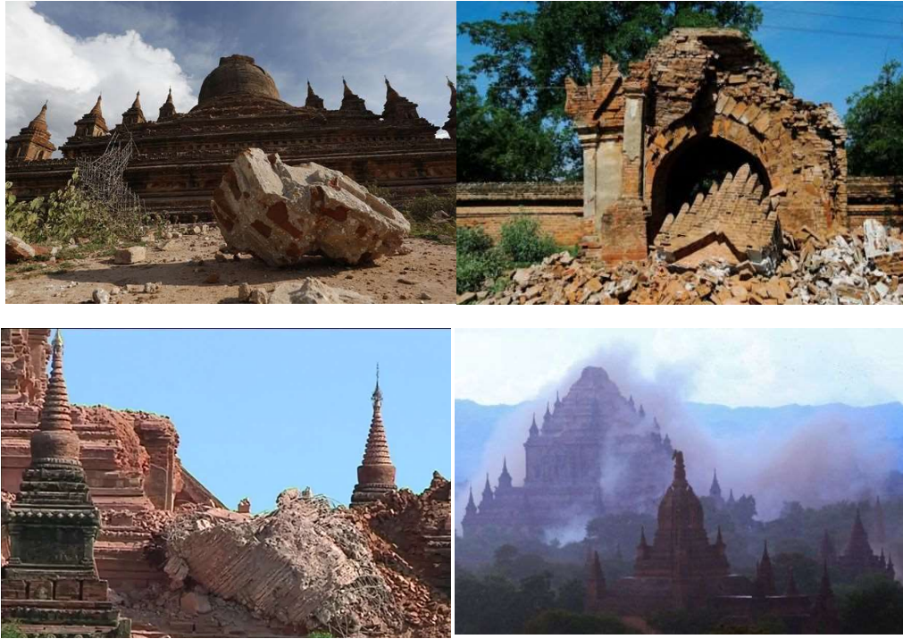
Figure (22, 23, 24, 25) The destruction of Ancient Bagan Temples and Pagodas Caused by (2016 Bagan Earthquake Source: Internet)
