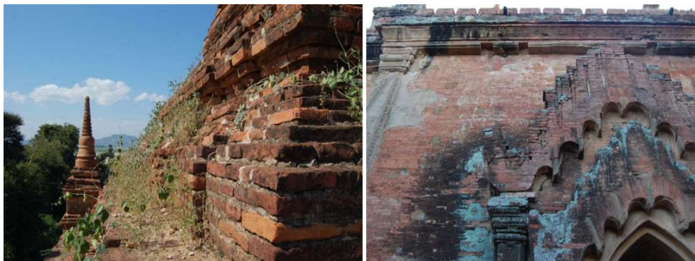
Figure (34) Damages Due to Vegetation and Microorganism
